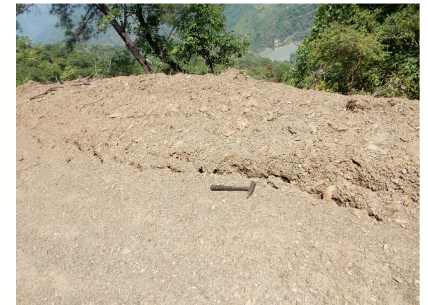
Development of Sympathetic Cracks at source region of a potential landslide at Ukhimath (Length of Hammer: 0.3m)
